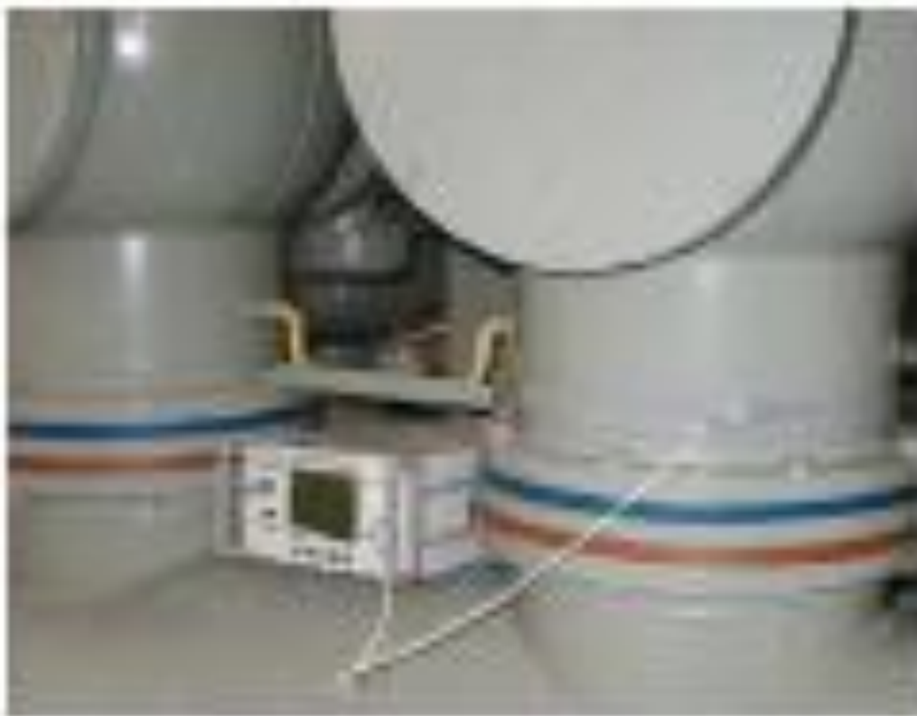
Figure 6c: Insulation monitoring on a 40 year old GIS by acoustic PD measurement
